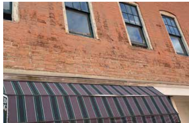
Example of masonry issues including spalling brick, peeling paint, and needed repointing.
