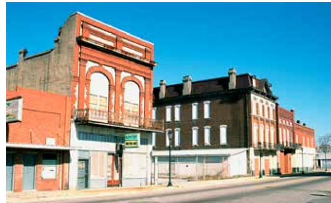
Photographs of existing conditions and issues are helpful tools in the analysis of a district.
