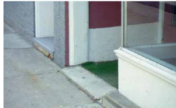
Many times a storefront entrance is already at grade, making accessibility feasible. However, other aspects of the entrance generally need to be verified and any changes should have minimal impact on existing historic materials or features.
