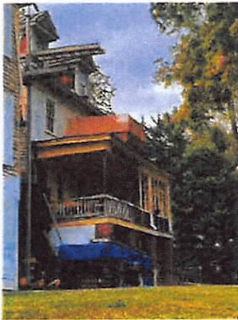
(Picture 12: Shows inadequate protection From elements and inadequate Structural supports on porch)
