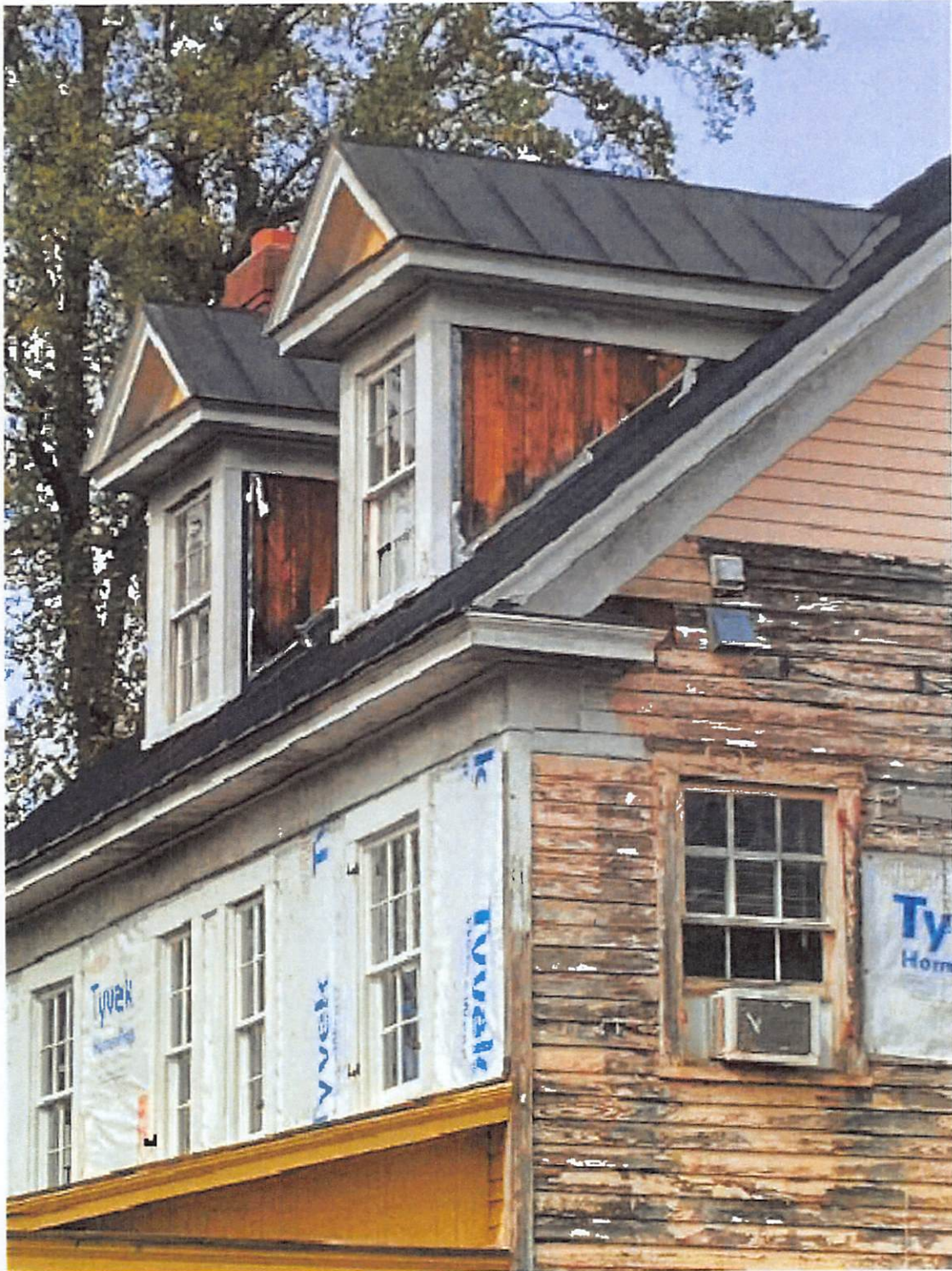
Picture 4: Shows exposure to the elements, wood rot, peeling paint, and inadequate roof drainage.
