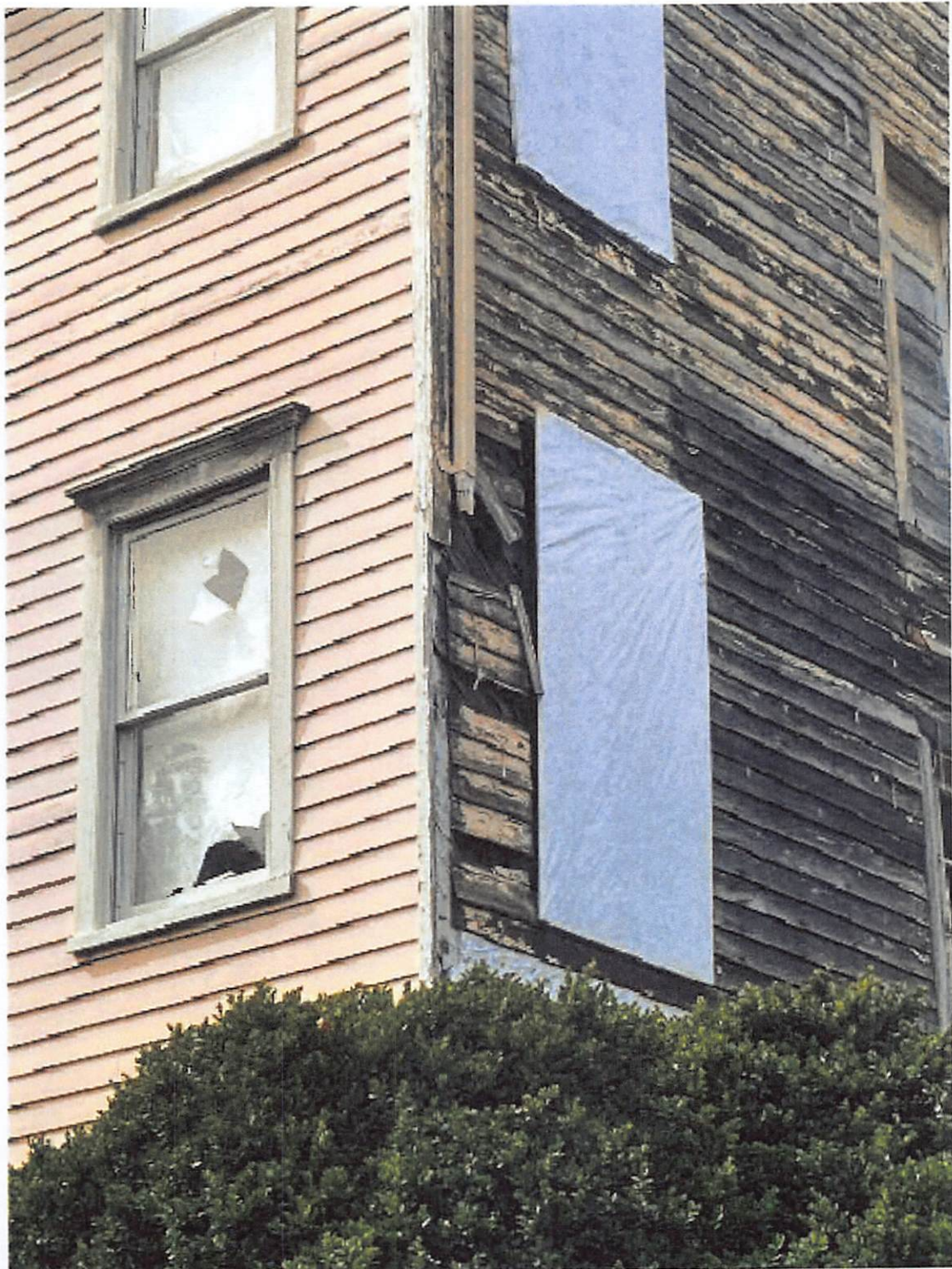
Picutre 9: Shows inadequate roof drainage, rotted wood and broken windows.
