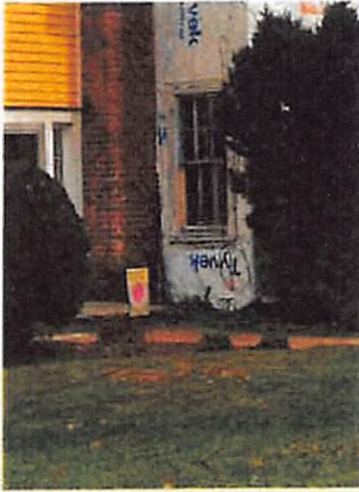
(Picture 13: Shows inadequate protection from elements)
