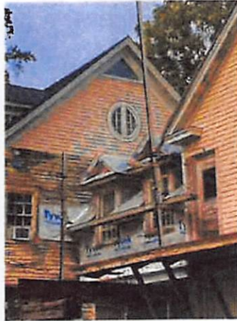
(Picture 2: Shows faulty structural supports, inadequate roofing and exposure to the elements)
