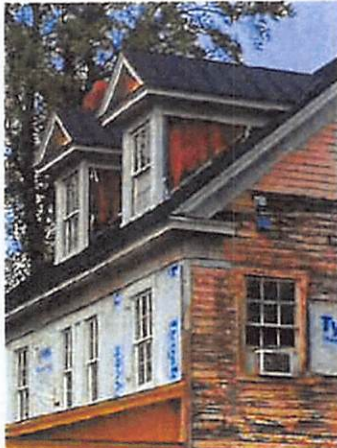
(Picture 4: Shows exposure to the Elements, wood rot, peeling Paint, and inadequate roof Drainage)
