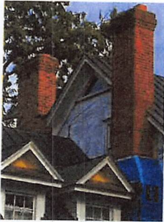
(Picture 7: Shows inadequate protection From the elements)
