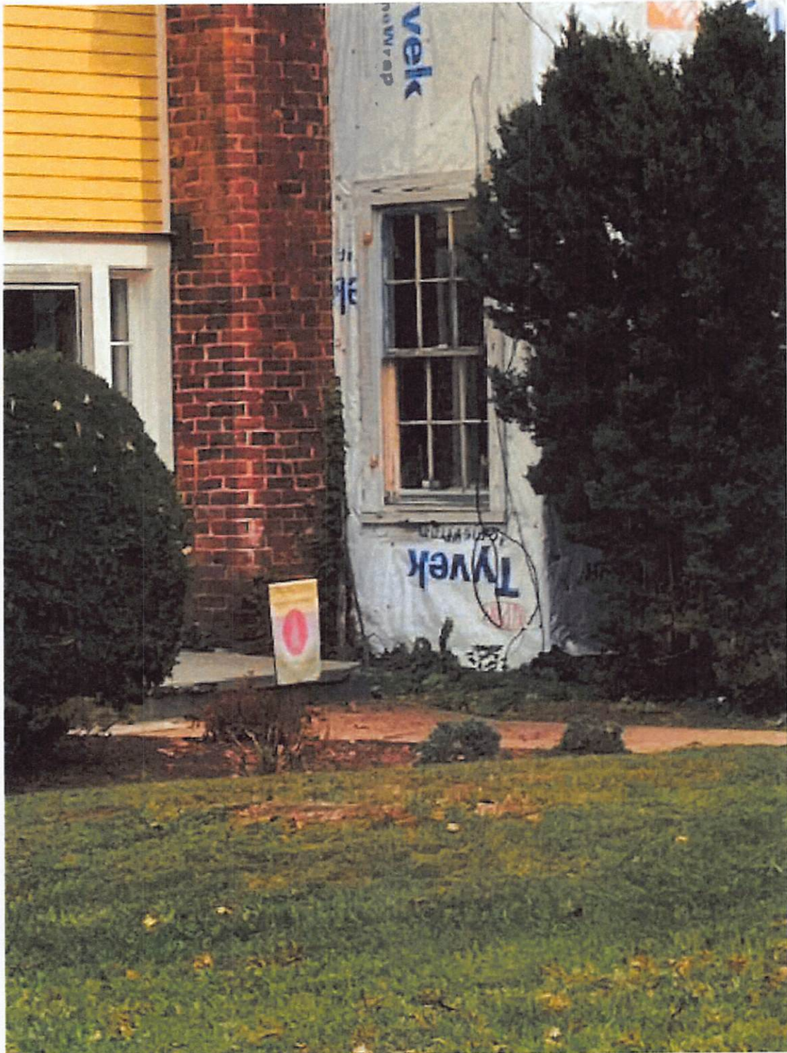
Picture 13: Shows inadequate protection from the elements.
