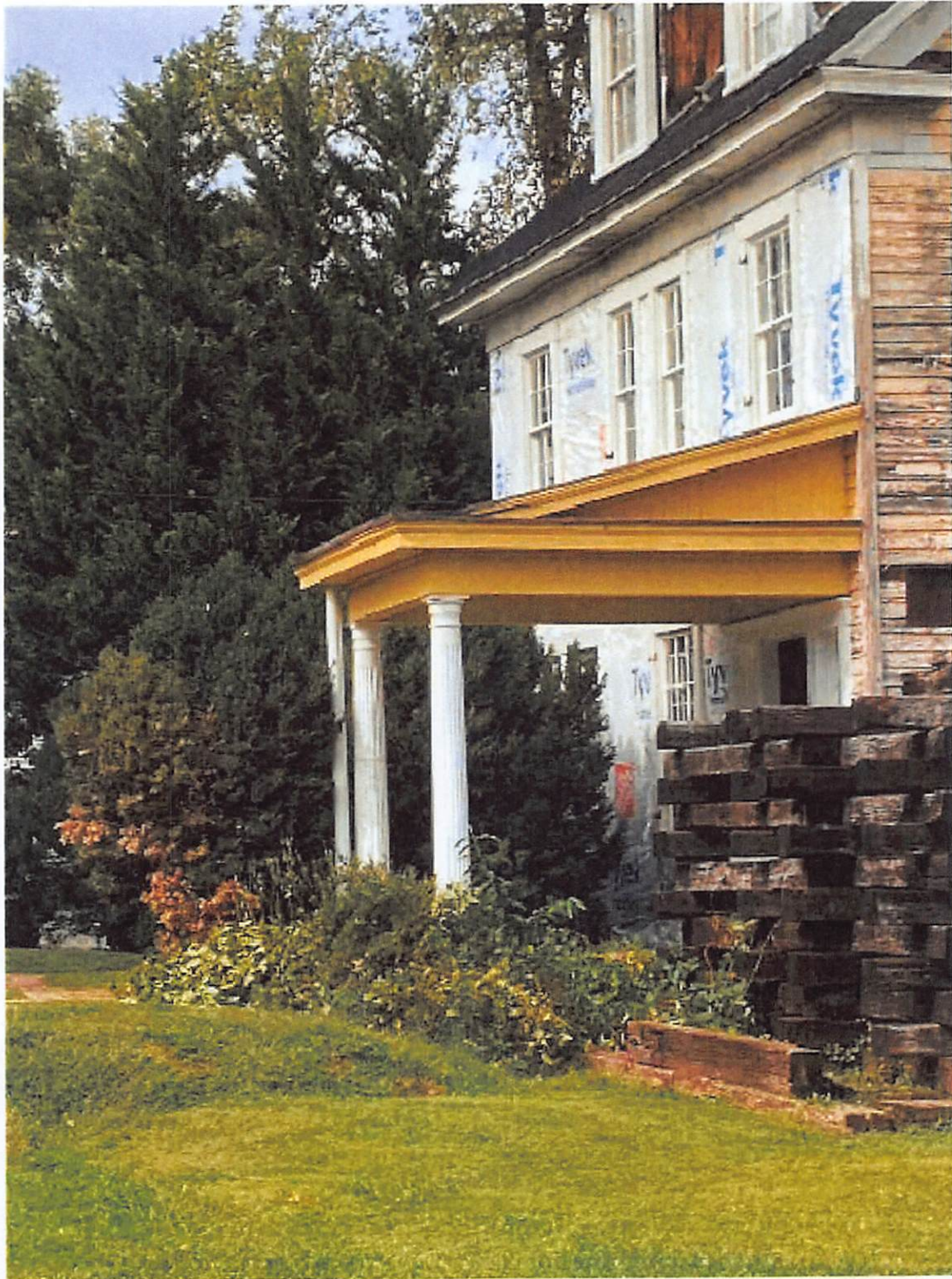
Picture 1: Shows exposure to the elements, rotted wood and inadequate roof drainage.
