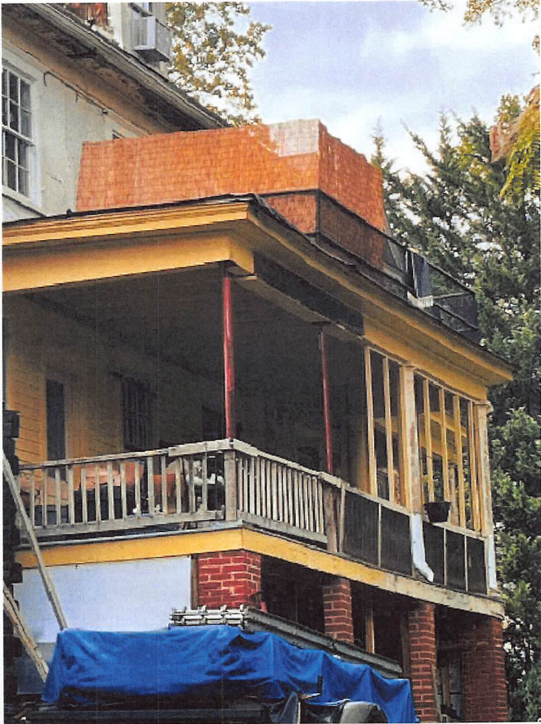
Picture 10: Shows inadequate structural supports, and inadequate protection from the elements.
