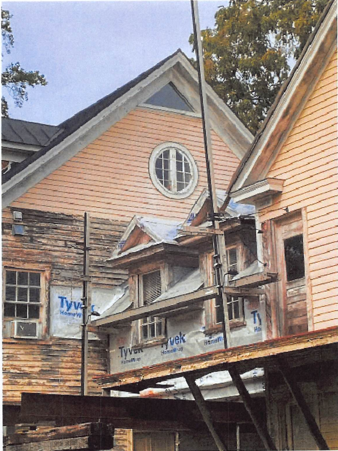
Picture 2: Shows faulty structural supports, inadequate roofing and exposure to the elements.
