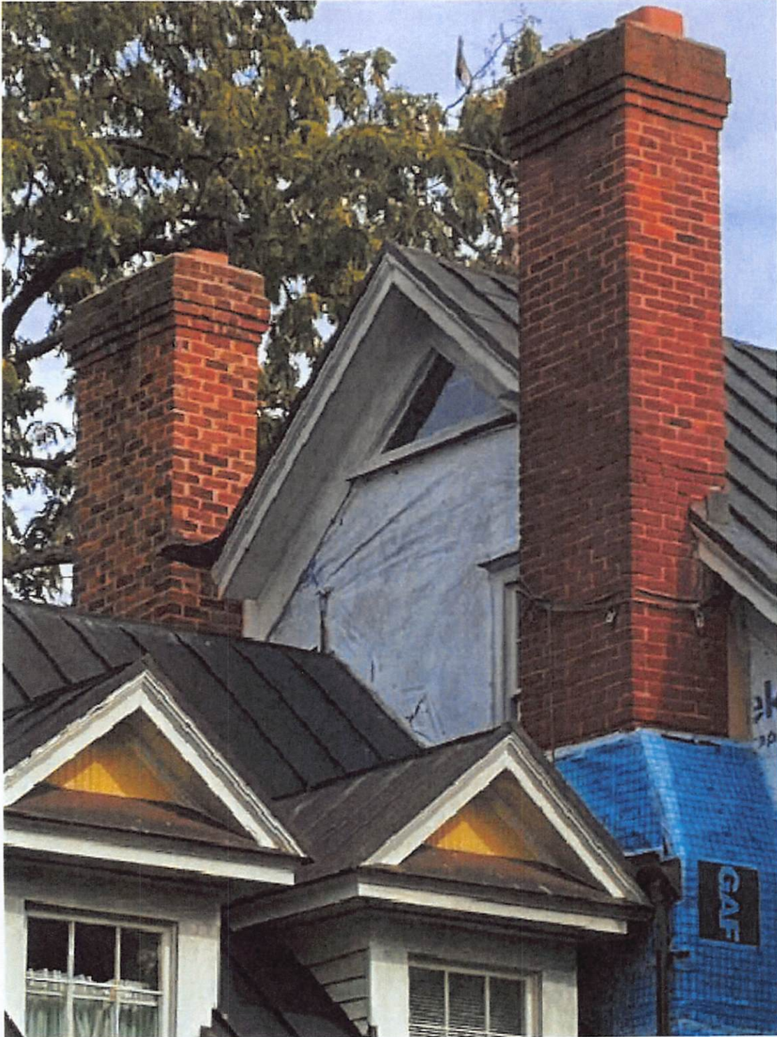
Picture 7: Shows inadequate protection from elements.
