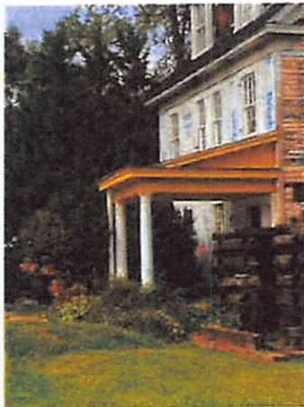
(Picture 1: Shows exposure to the Elements, rotted wood and inadequate roof drainage)
