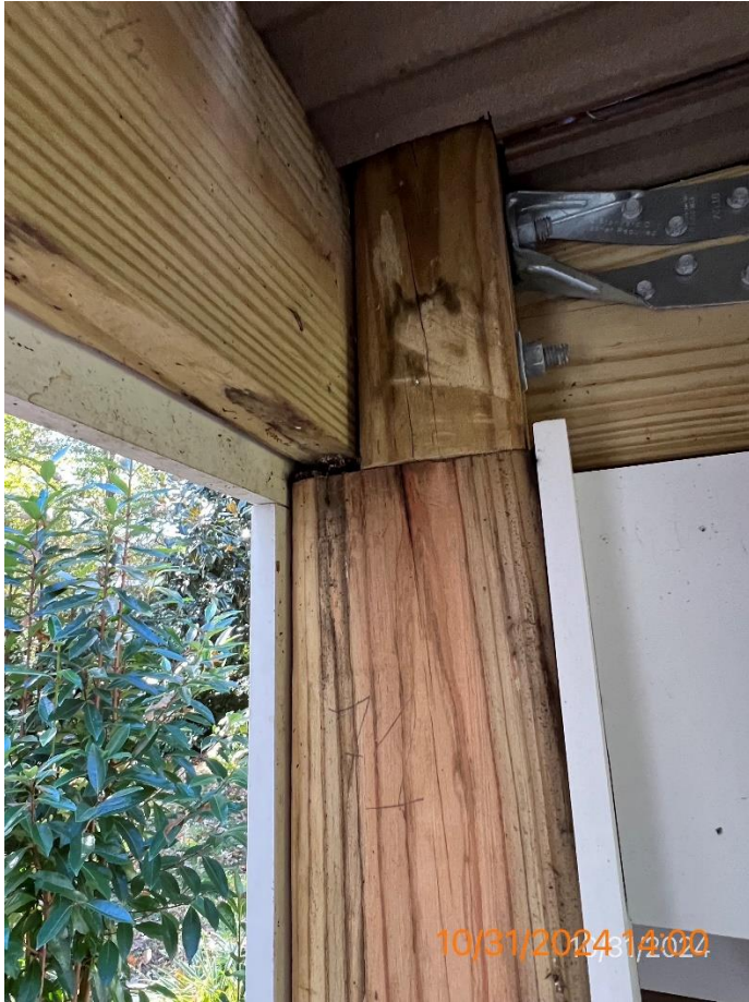
Figure 12 - Close-up of the top section of the support post that is rotted under deck - Guard Post Connections and Post to Beam connection violation
