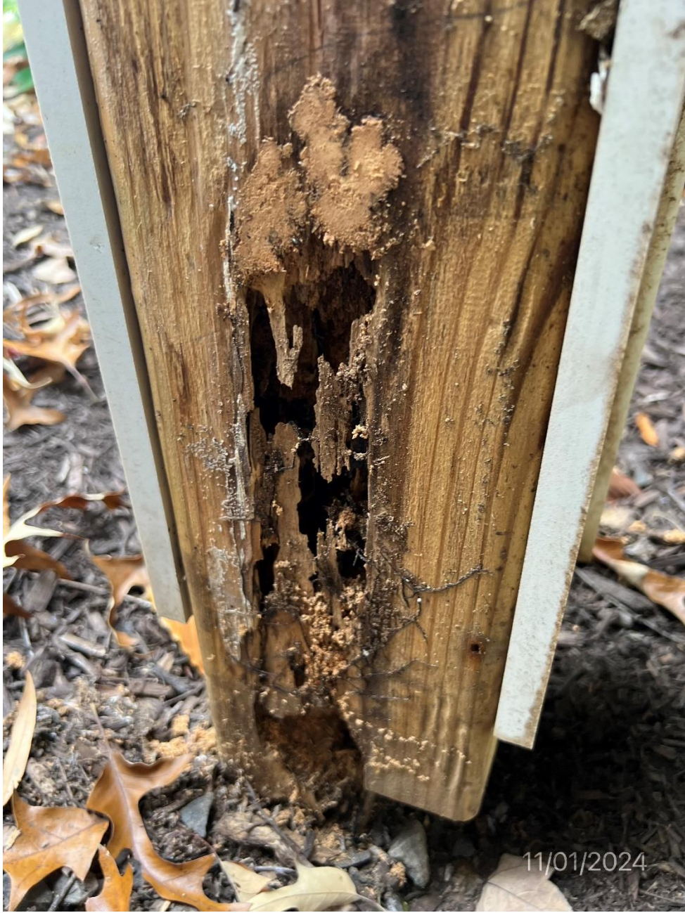
Figure 10 - Another close-up of rotting post
