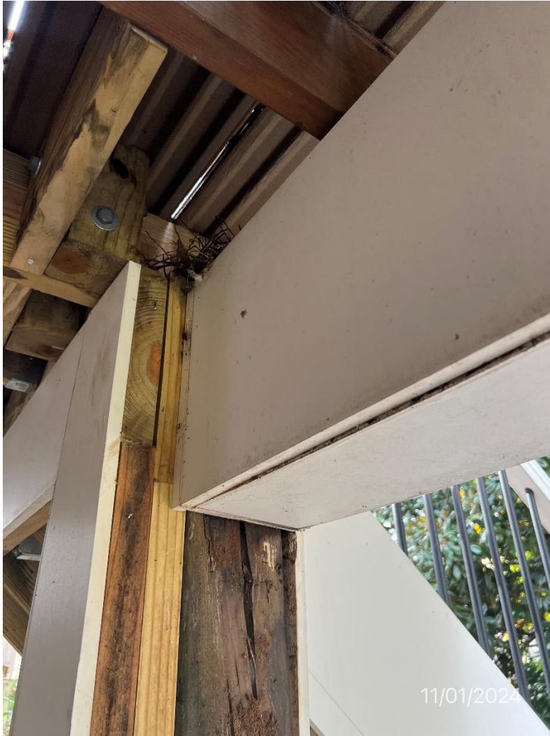
Figure 15 - Close up of top section closest to patio post to beam connection not correctly installed per violation FFC listing
