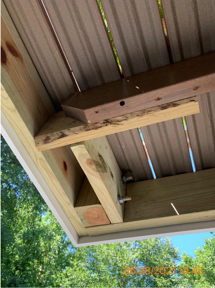
Figure 20 - New deck extensions (blocking) are not per code. Need to be a min. 3 to 1 ratio at deck cantilever. Same for each across the underside of deck
