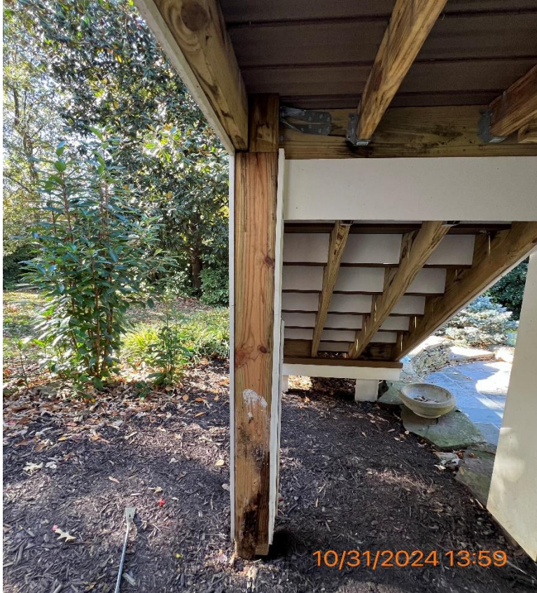
Figure 6 - Full view of incorrectly notched post with PVC removed and post to beam connection pg 14 _ figure 18
