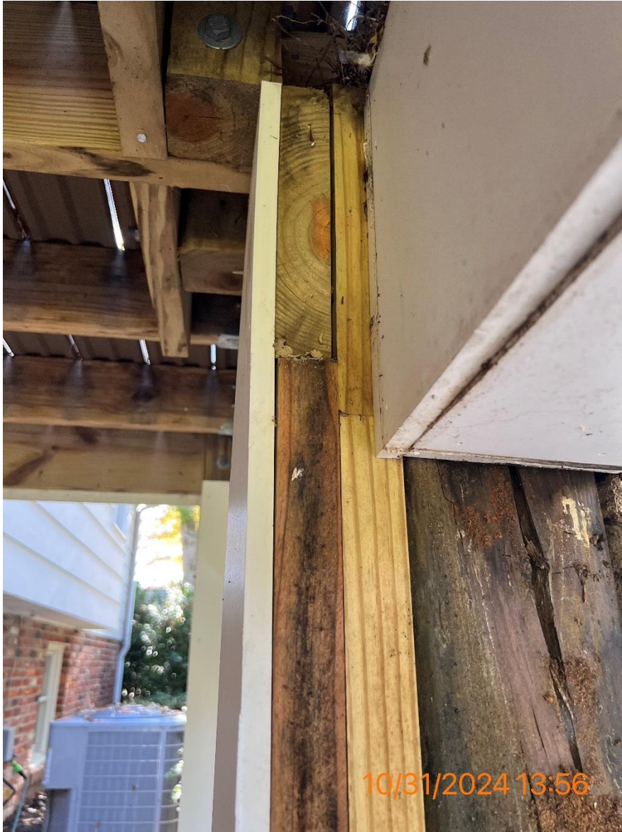
Figure 14 - Original post with alterations with rot and cracking under white PVC support beam that runs across the front of deck
