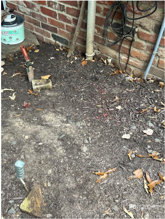
Figure 4 - Original cut down post photos location under upper right landing where new deck was attached to cantilever
