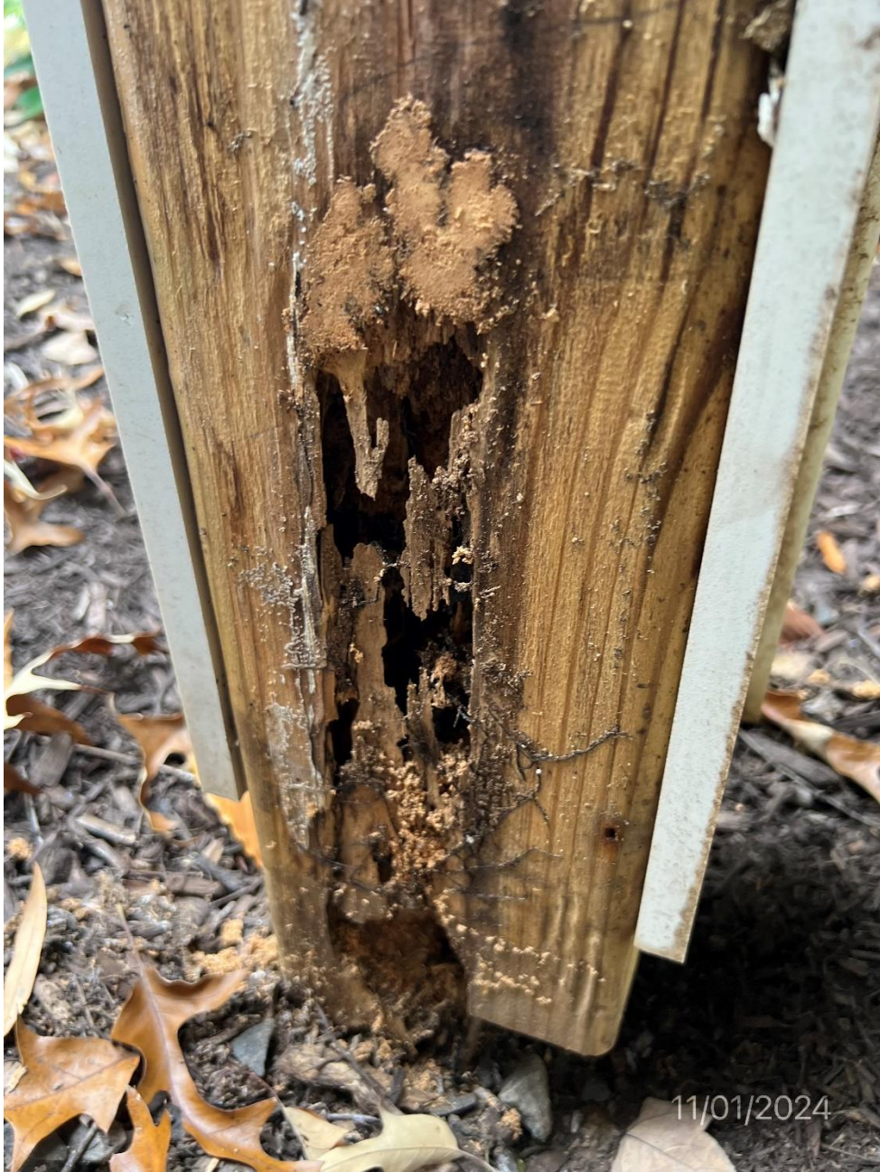
Figure 10 - Another close-up of rotting post
