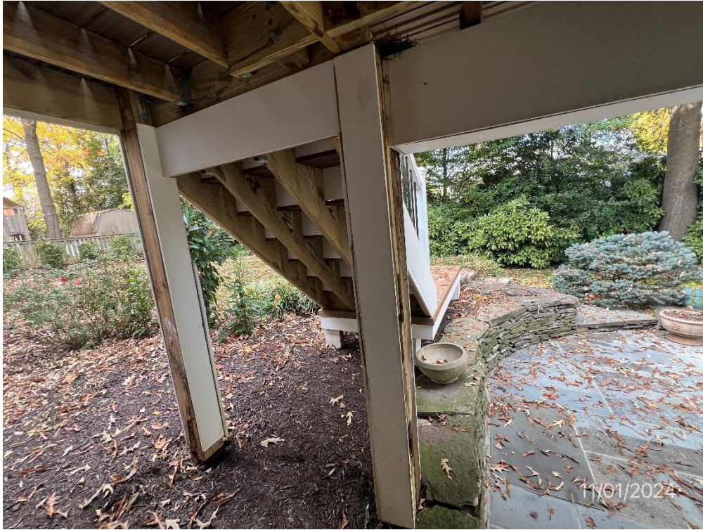
Figure 5 - Underside of the two existing reused posts with rot on both and alterations to one closest to patio
