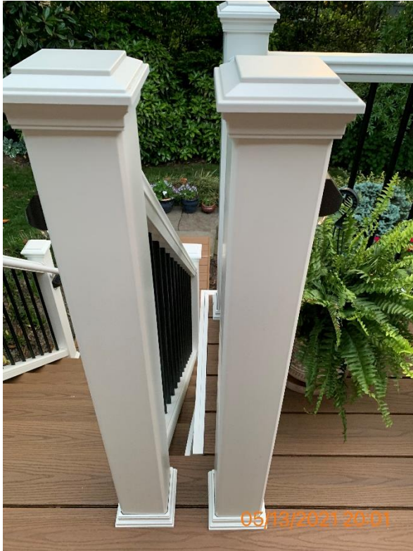
Figure 21 - Spacing between guard post at top of stairs is more than 4 inches. Need to secure stair treads properly
