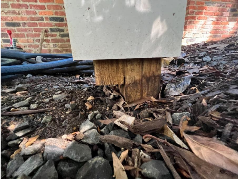
Figure 8 - Close up of back right post under stairs that was incorrectly notched violation
