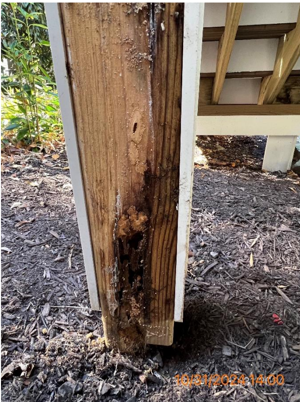
Figure 9 - Rotting post that was incorrectly notched - Post to beam connections at top and bottom landings not attached correctly, FFC Post to Beam connection pg.14_ figure18
