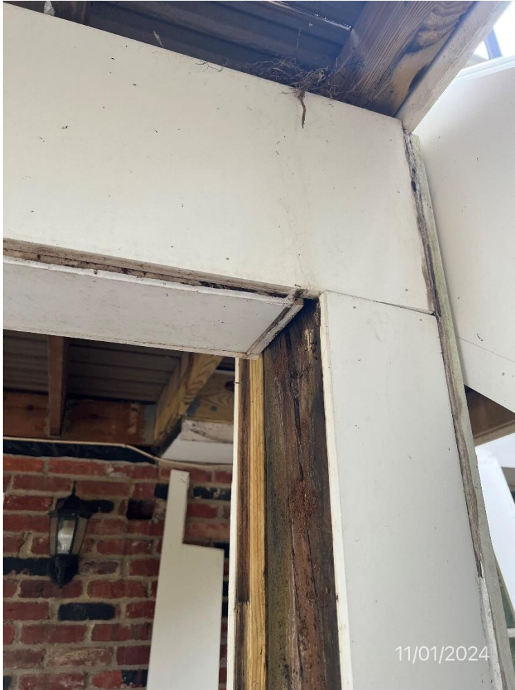
Figure 17 - Another view of the post closest to the patio with support beam to its left that is open on the top where debris and water are collecting and effecting the top post's cracking and deterioration
