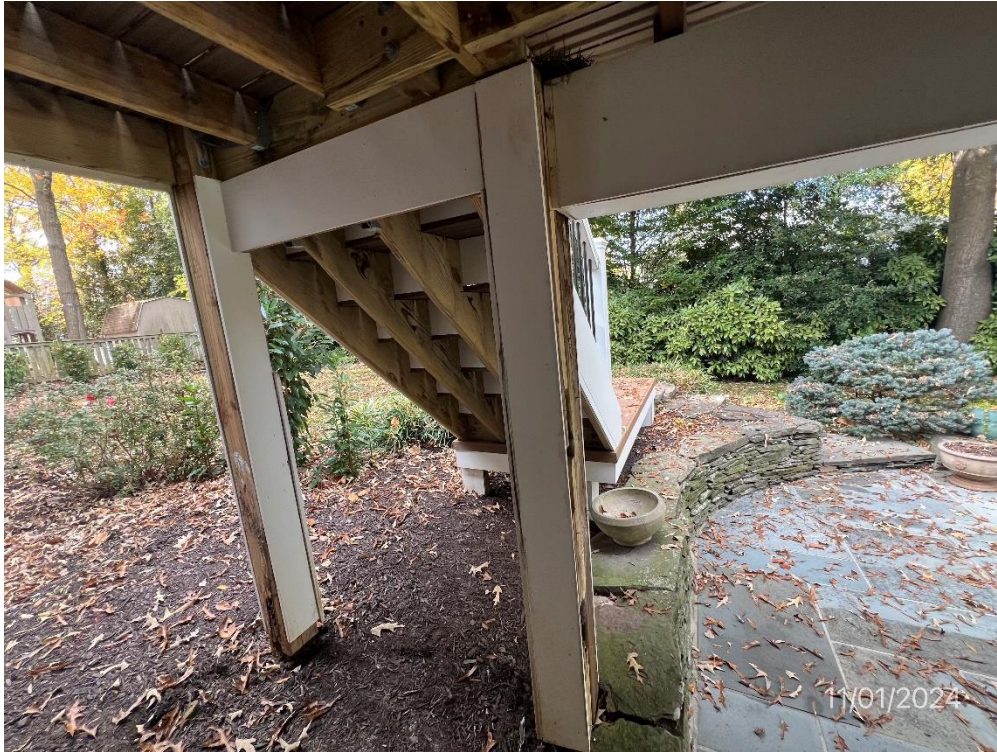
Figure 5 - Underside of the two existing reused posts with rot on both and alterations to one closest to patio
