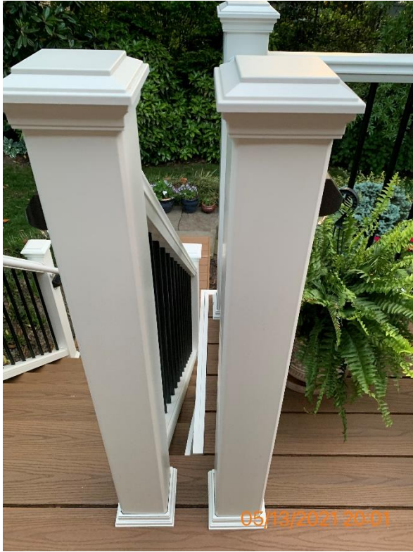
Figure 21 - Spacing between guard post at top of stairs is more than 4 inches. Need to secure stair treads properly
