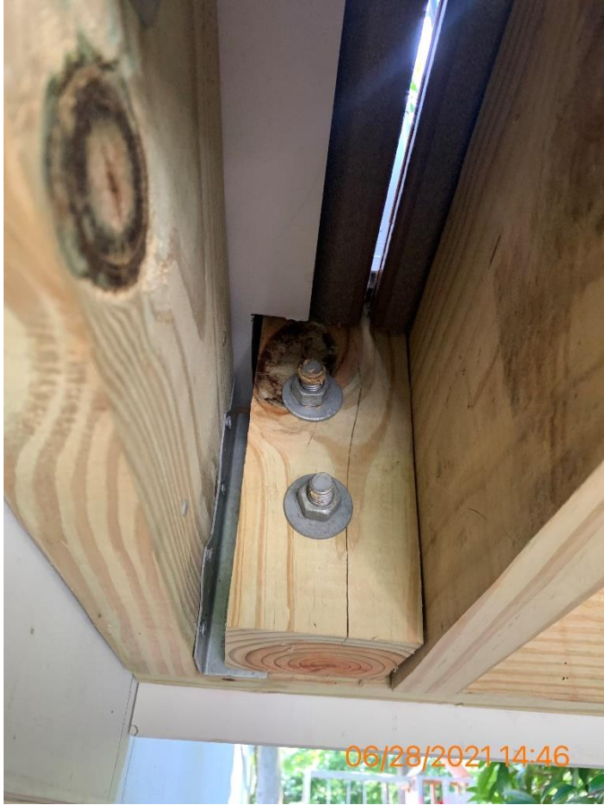
Figure 19 - All Guard Post connections need to be constructed per FFC Detail_Guard Post Connections Pages 20 21 and 24 Figures 37 38 and 40
