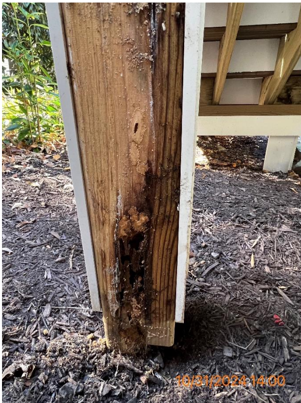
Figure 9 - Rotting post that was incorrectly notched - Post to beam connections at top and bottom landings not attached correctly, FFC Post to Beam connection pg.14_ figure18
