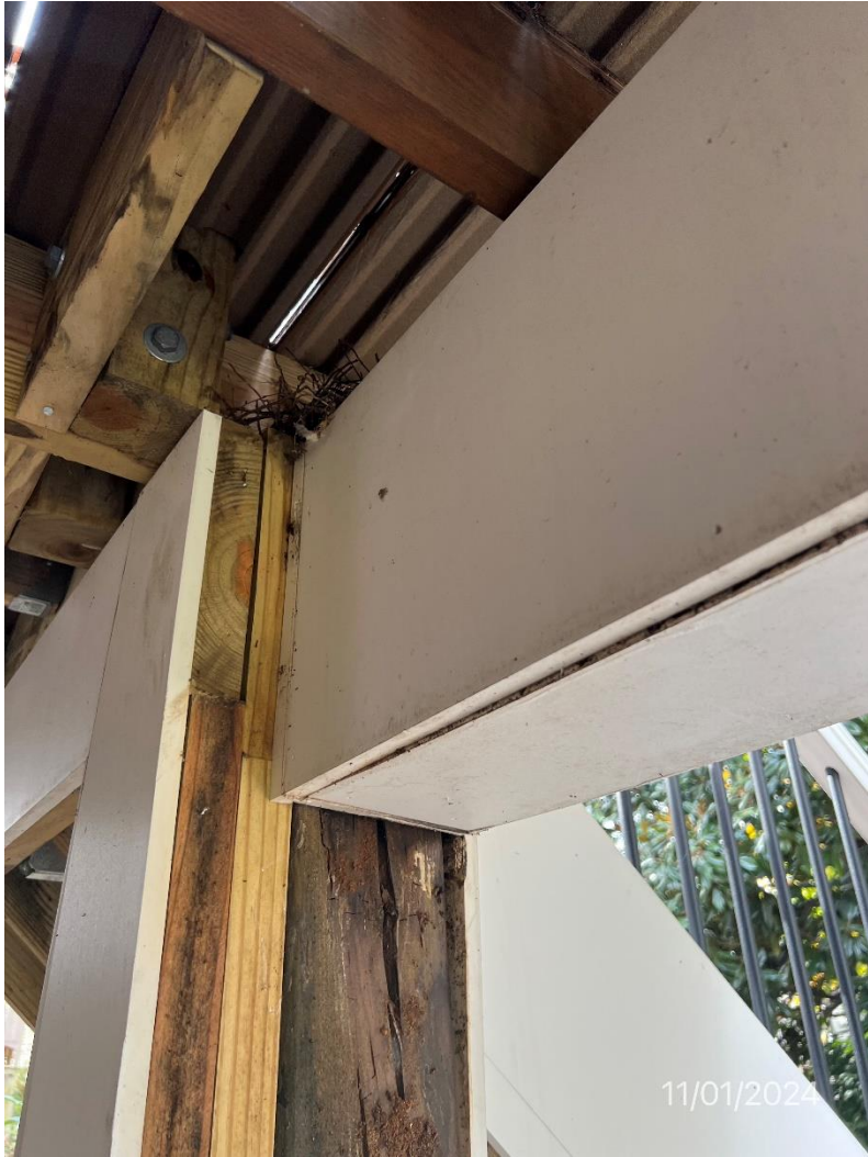
Figure 15 - Close up of top section closest to patio post to beam connection not correctly installed per violation FFC listing
