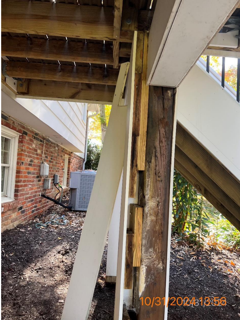
Figure 11- Original altered post with PVC removed. Top section left side where block is left unsupported - Post to beam connections violation
