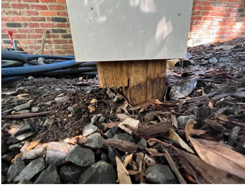
Figure 8 - Close up of back right post under stairs that was incorrectly notched violation
