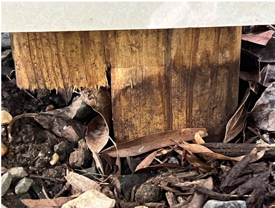
Figure 7 - Facing deck back right post under stairs with incorrect notch violation
