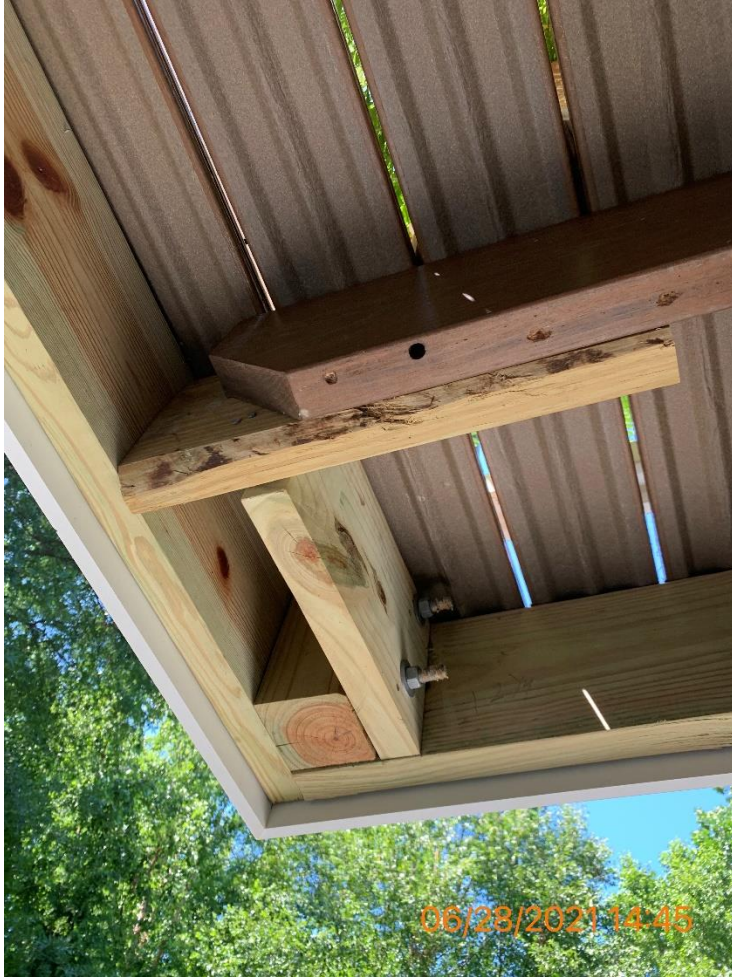
Figure 20 - New deck extensions (blocking) are not per code. Need to be a min. 3 to 1 ratio at deck cantilever. Same for each across the underside of deck
