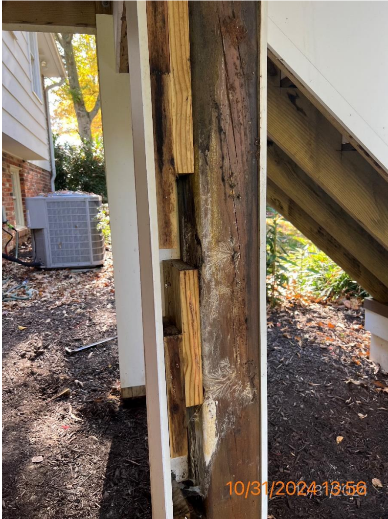
Figure 16 - Close up of top section closest to patio post to beam connection not correctly installed per violation FFC listing
