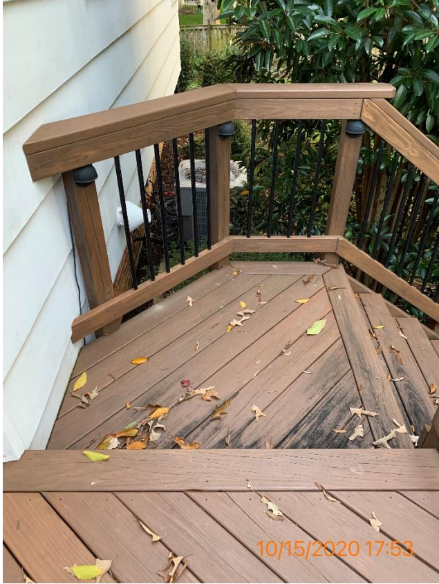
Figure 24 - Prior deck photo provided for context of the original upper landing which had two support beams cut down. Landing eliminated by GLK and instead attached deck to cantilever
