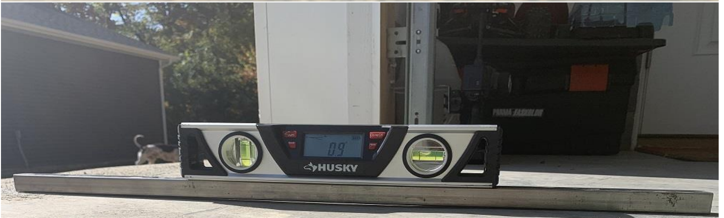
Attached garage image 1 taken 10/20/2020 by Monica Davis @ 2:43 PM level setting on 24" steel bar will show negative .9% toward the back wall.
