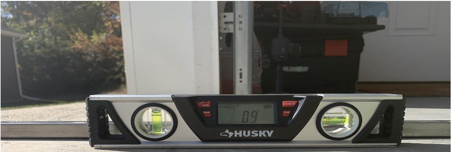
Attached garage image 1 taken 10/20/2020 by Monica Davis @ 2:44 PM level setting on floor will show negative .9% toward the back wall.
