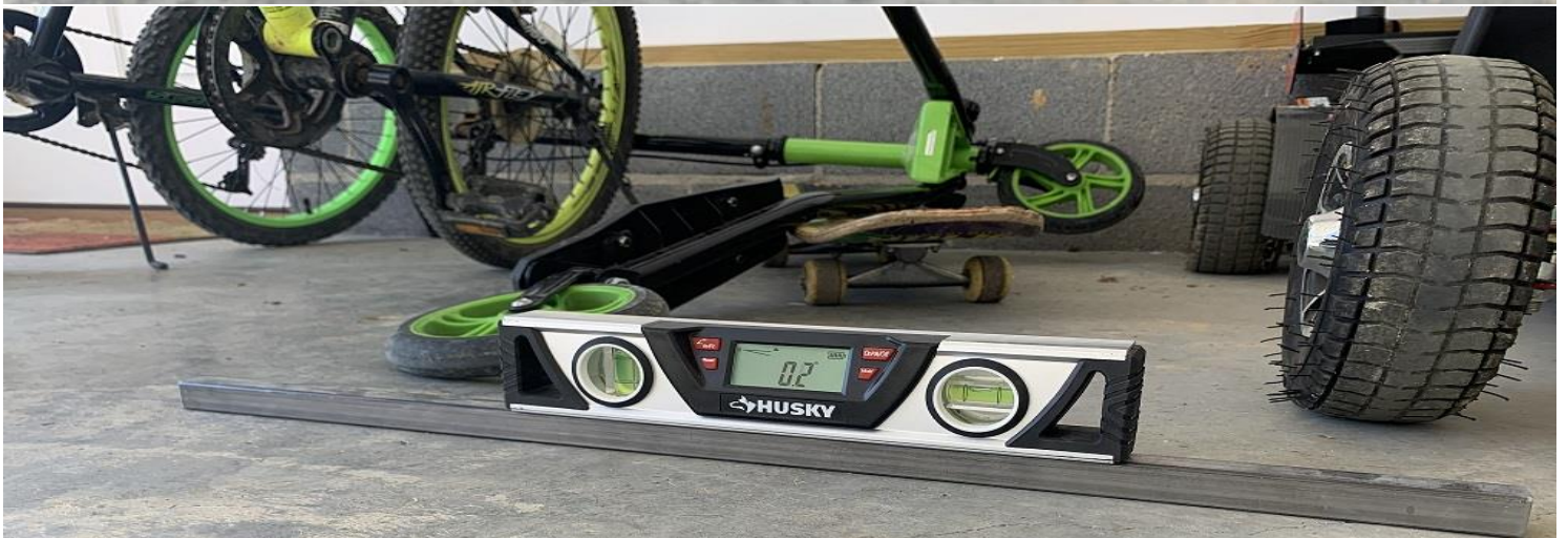
Attached garage image 4 taken 10/20/2020 by Monica Davis @ 2:55 PM level setting on 24" steel bar will show negative .2% toward the back wall.
