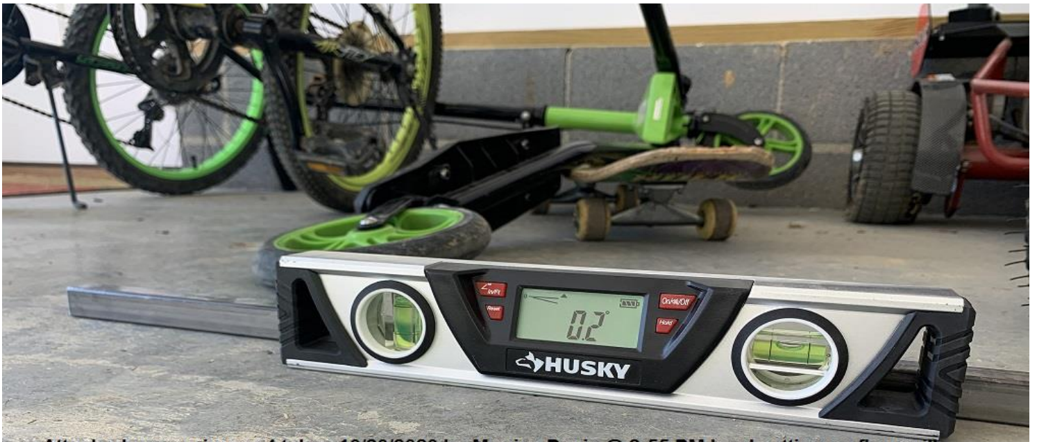
Attached garage image 4 taken 10/20/2020 by Monica Davis @ 2:55 PM level setting on floor will show negative .2% toward the back wall.
