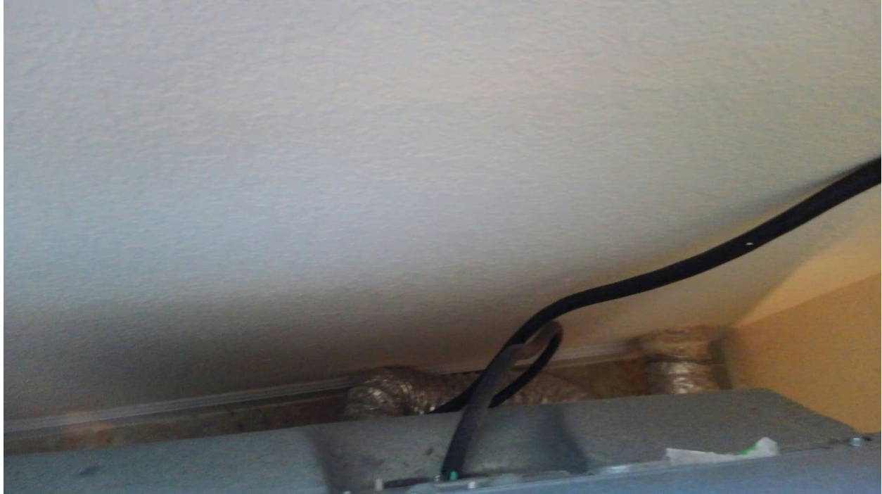
Image 12, Showing outlet hose arrangement behind clothes dryer.
