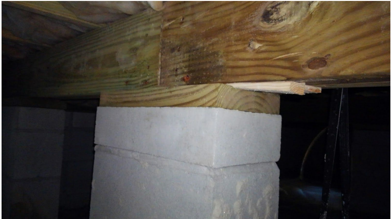
Image 15, Showing non treated, non uniform thickness wood being used to shim beam at crawl space.
