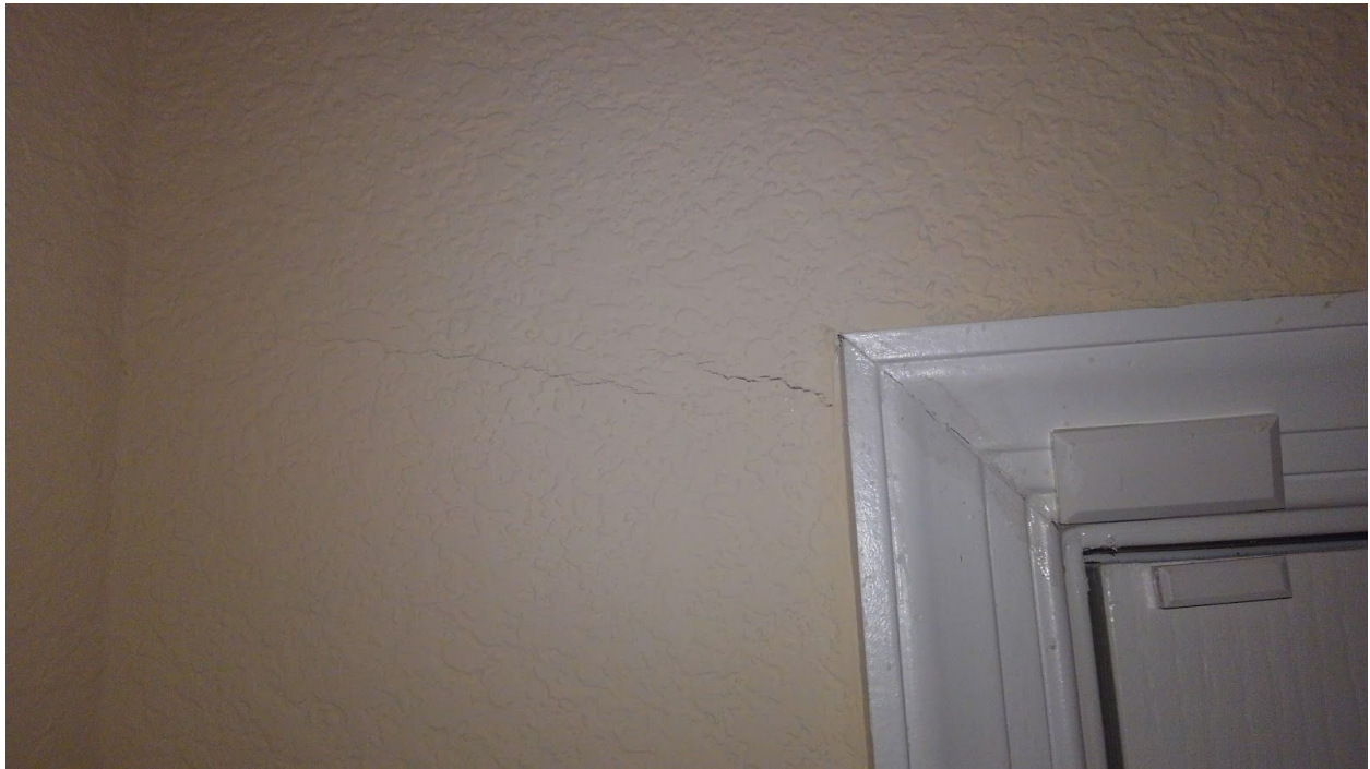
Image 10, Showing typical drywall cracking at doorway.
