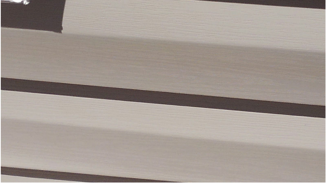
Image 5, SHowing Dutch lap siding that has been face nailed through the weep holes.
