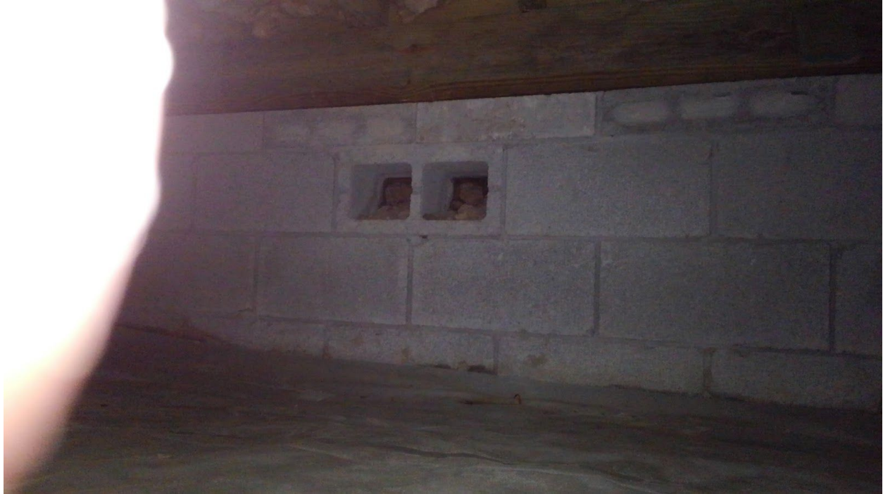
Image 16, Showing blocked vent at front of structure in crawl space.
