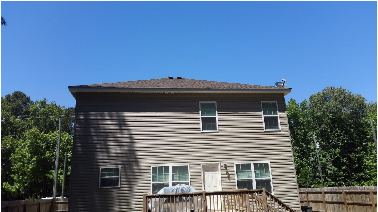
Image 2, Showing lifting of shingles at left hip.
