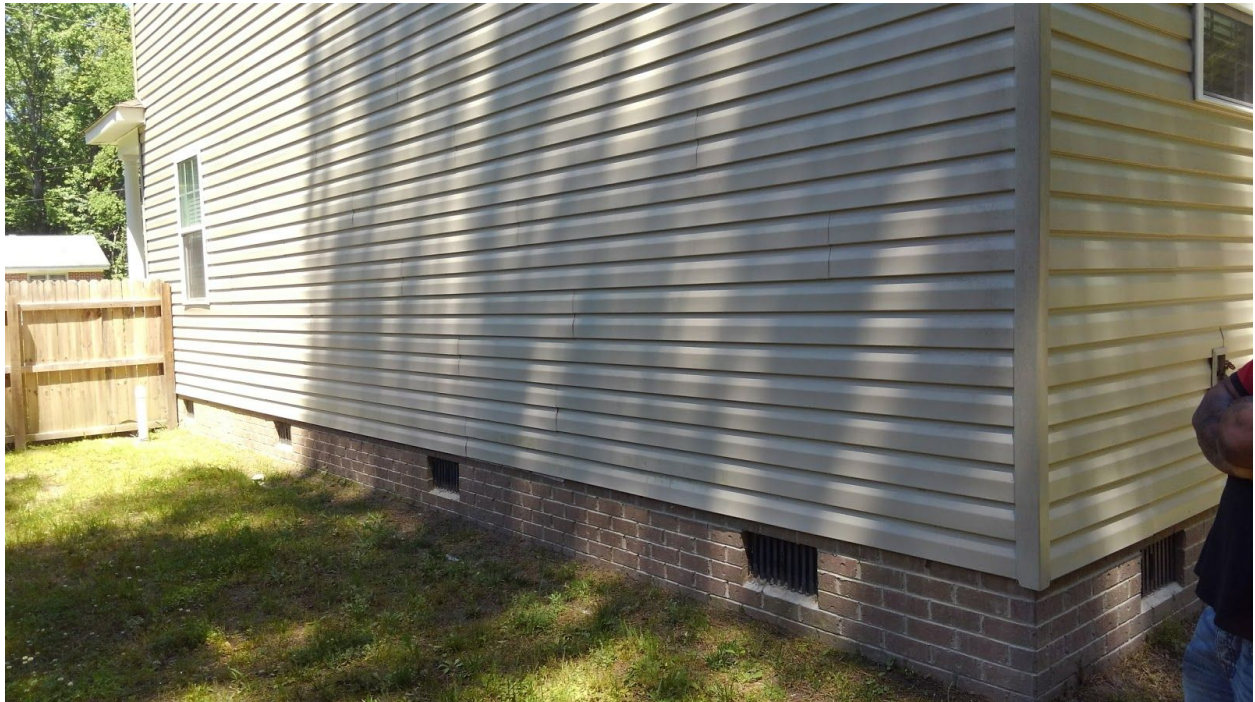
Image 4, Showing side wall of home where face nails have been installed through siding weep holes.
