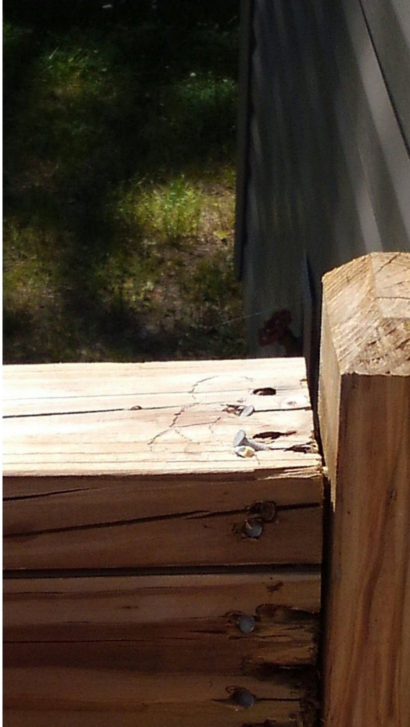
Image 17, Showing degraded deck railing from over nailing.
