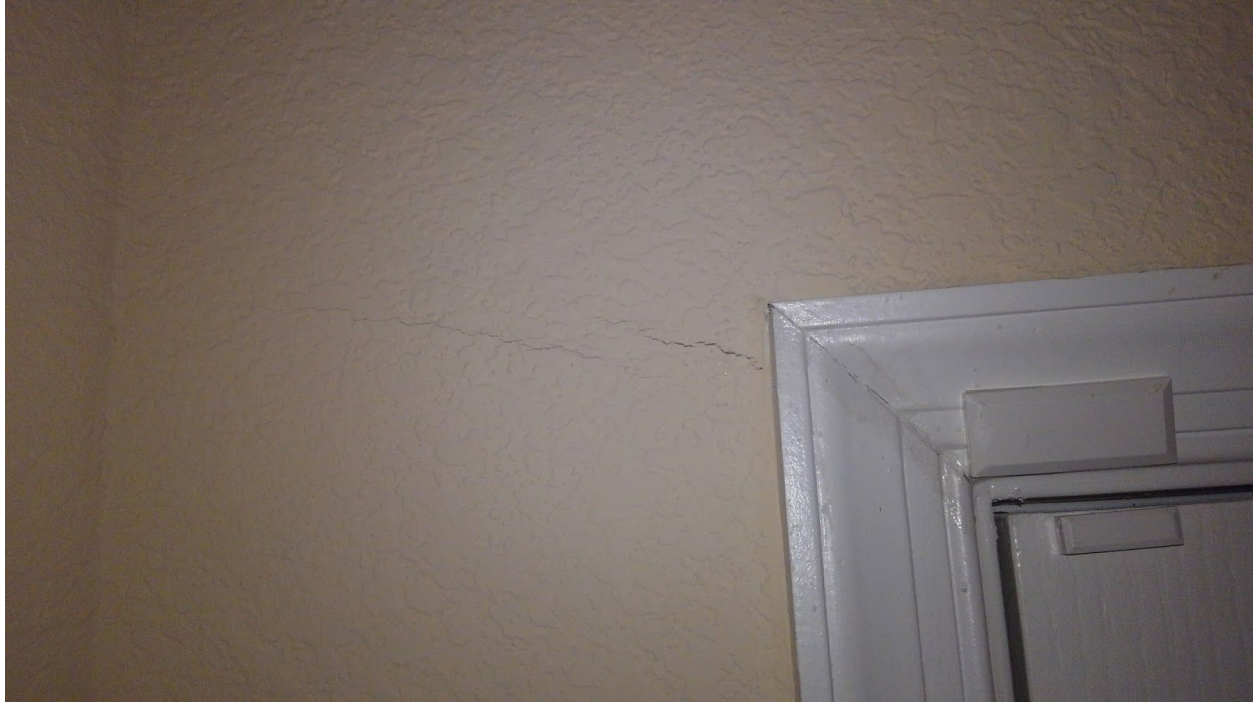
Image 14, Showing cracking at garage door.
