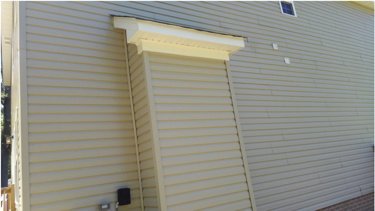
Image 6, Showing the opposing side wall where face nails have been used to secure siding.
