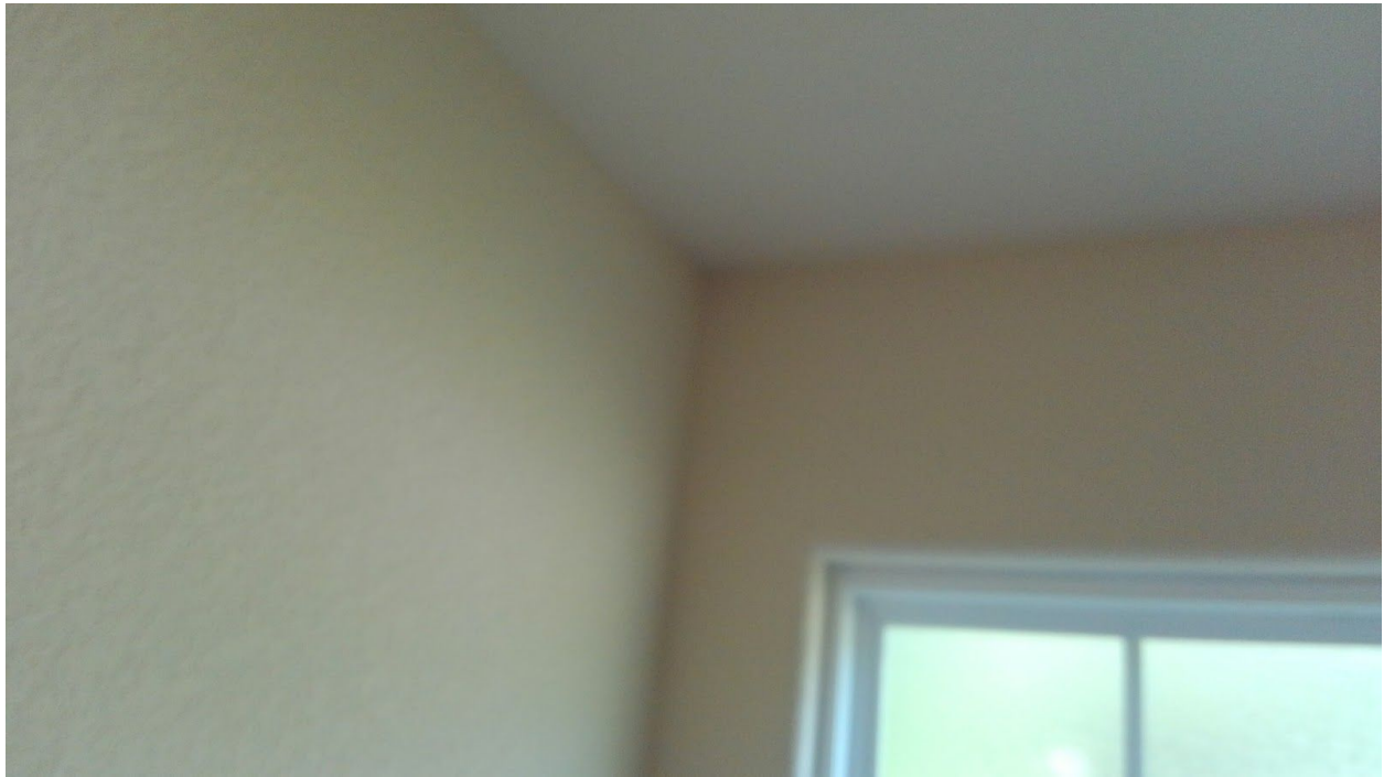
Image 12, Showing further evidence of drywall cracking at ceiling.
