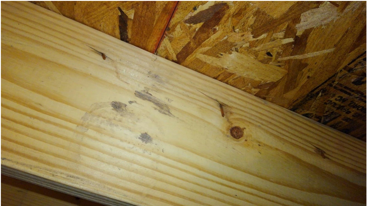
Image 9, Showing exposed nail end with evidence of rust, in unconditioned attic.
