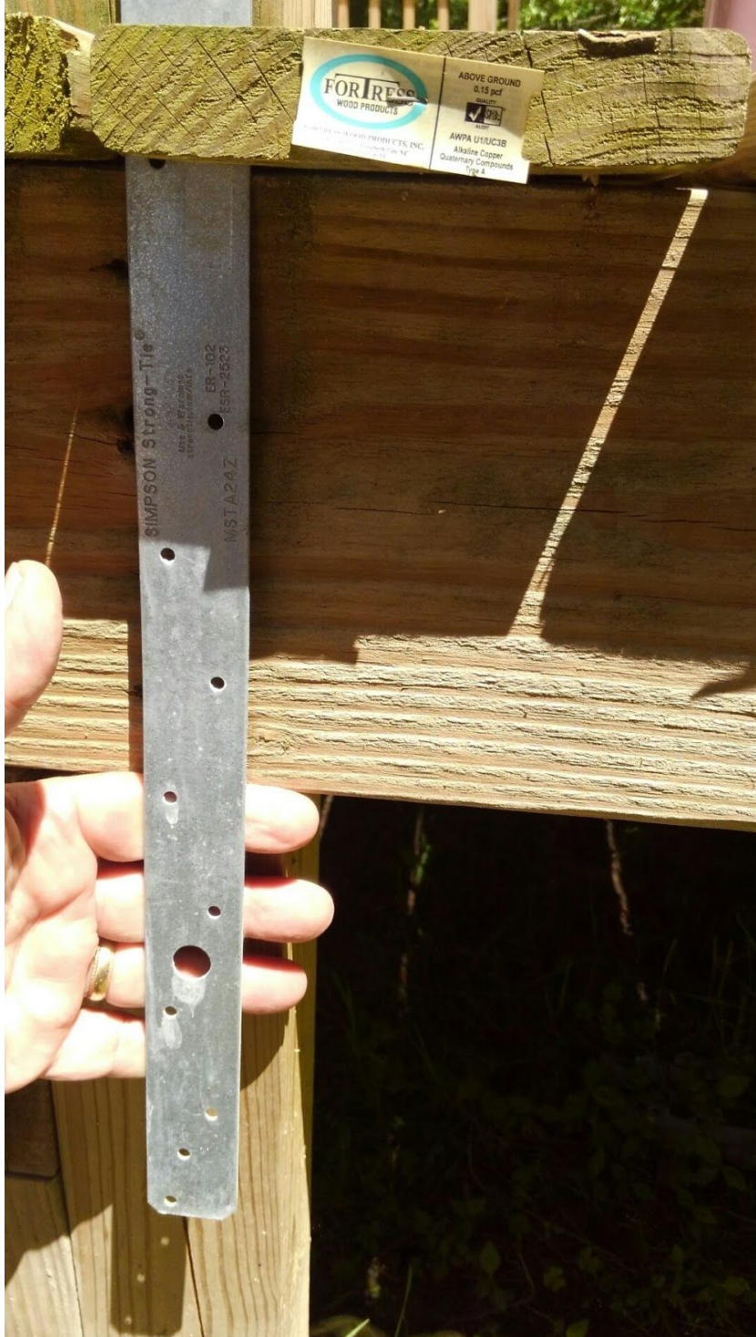
Image 18, Showing missing connector nails at deck railing post.
