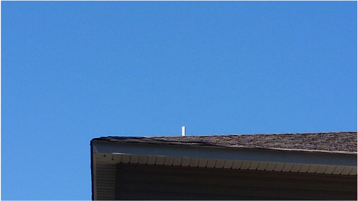
Image 3, Close-up of lifting shingles at left hip.
