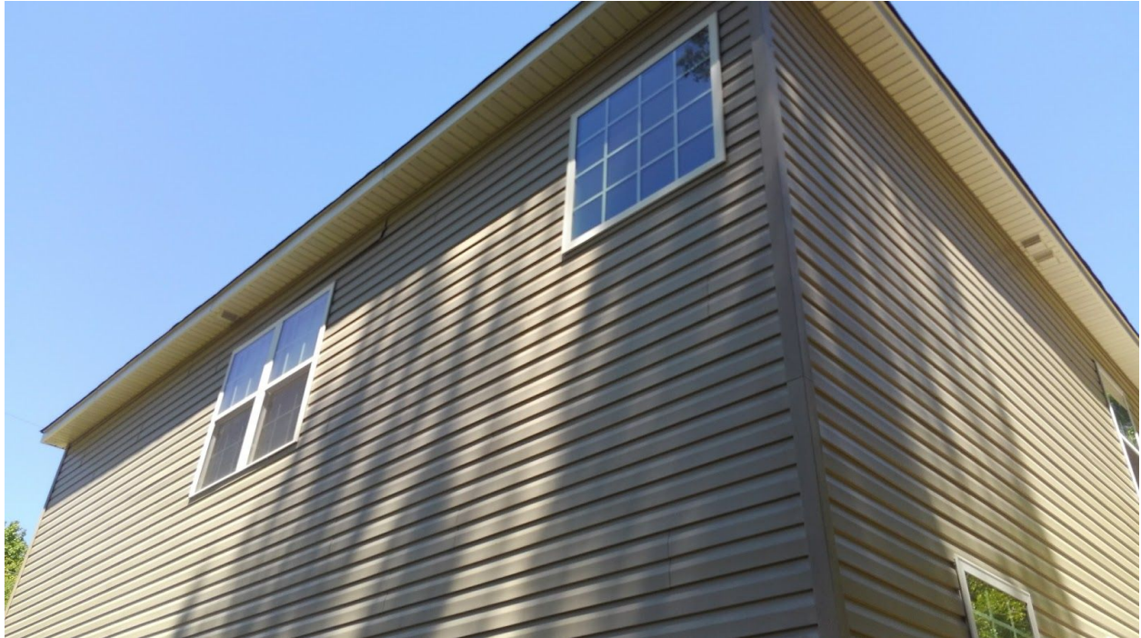
Image 1, Showing lack of gutters or downspouts.
