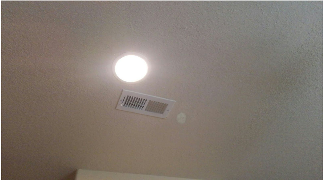
Image 13, Showing ceiling damage at pantry closet.
